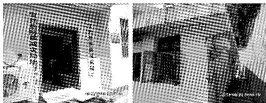
图17 宝兴县防震减灾局办公楼严重破坏 Fig. 17 Damaged office for Baoxing Bureau of Earthquake Mitigation
